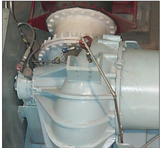
Close-up view showing pump, casing area and piping connection.
